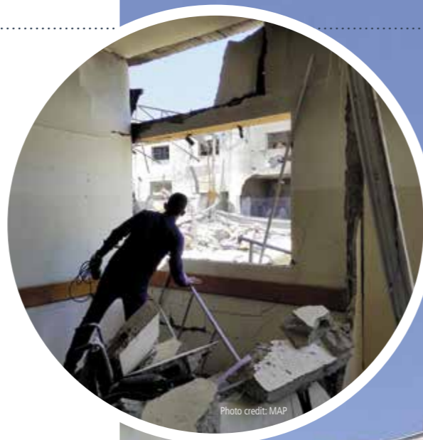
Gaza's Al-Rimal Clinic in the Ministry of Health's headquarters, which was severely damaged during Israel's military offensive in May 2021.
